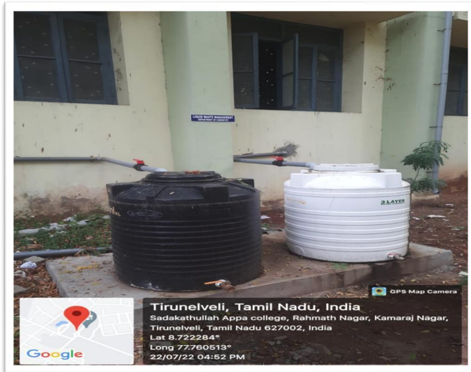
Liquid Waste Management Tank: Department of Chemistry
