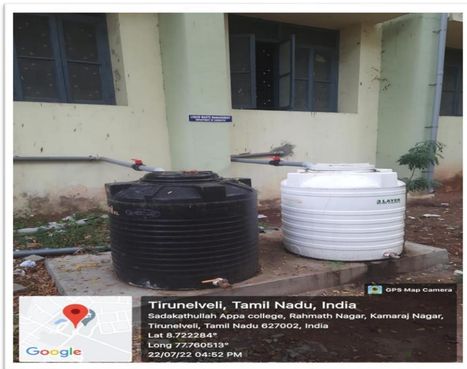
Liquid Waste Management Tank: Department of Chemistry
